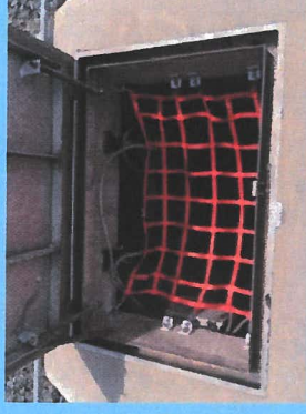
Fall Protection Open Hatches
